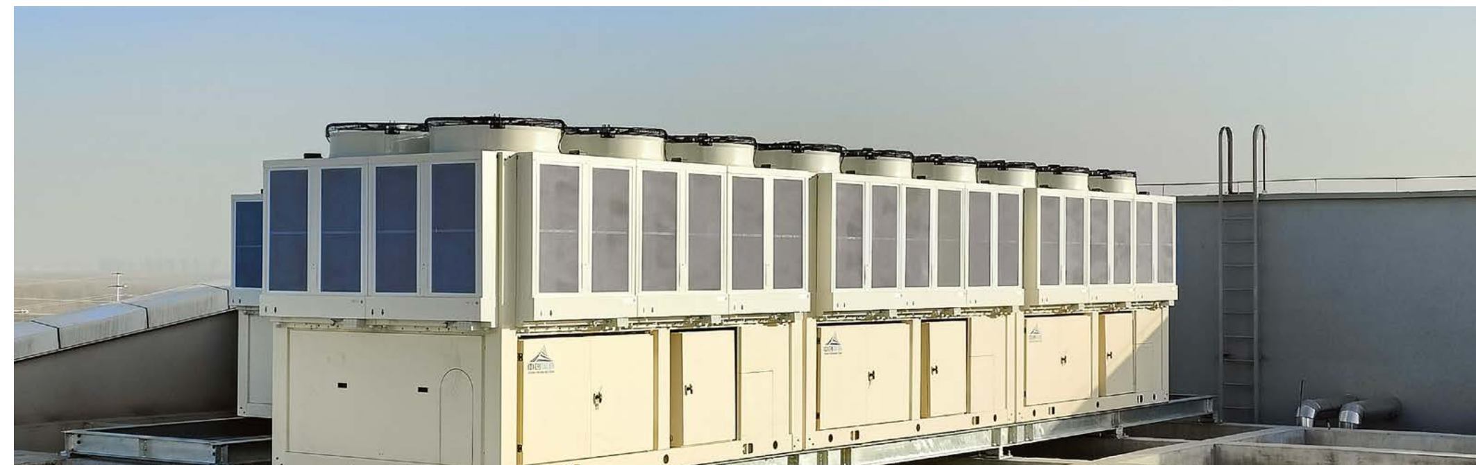
Evaporative Cooling System
