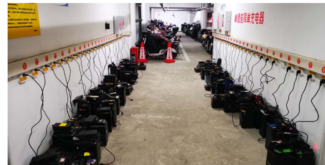
Electric Bicycle Charging Piles
