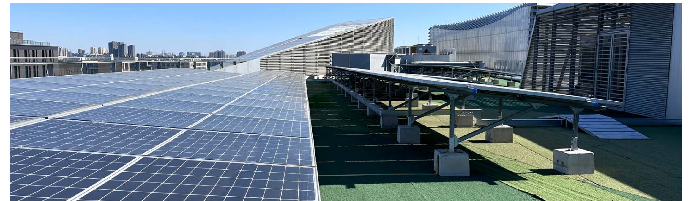
PV System of Weibo Data Center
